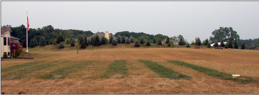
Figure 2. Unusually green turfgrass stripes represent a stressed septic system that is failing or likely to fail during wetter months or when the system receives high wastewater flows.
